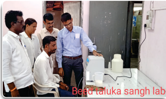
Installation of EMAT Advance at Beed Taluka Sahakari Duddh Utpadak Sangh Ltd, Maharashtra
