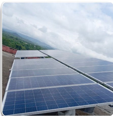
8kWP SPV Power Plant installed at Piplantri Village for powering Water Pumping Systems
